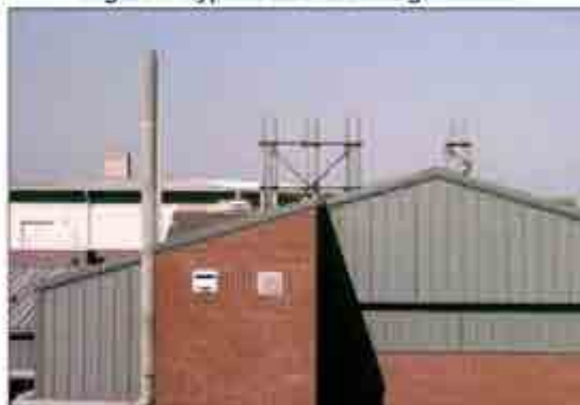
Figure 9 Typical LEV discharge stacks
