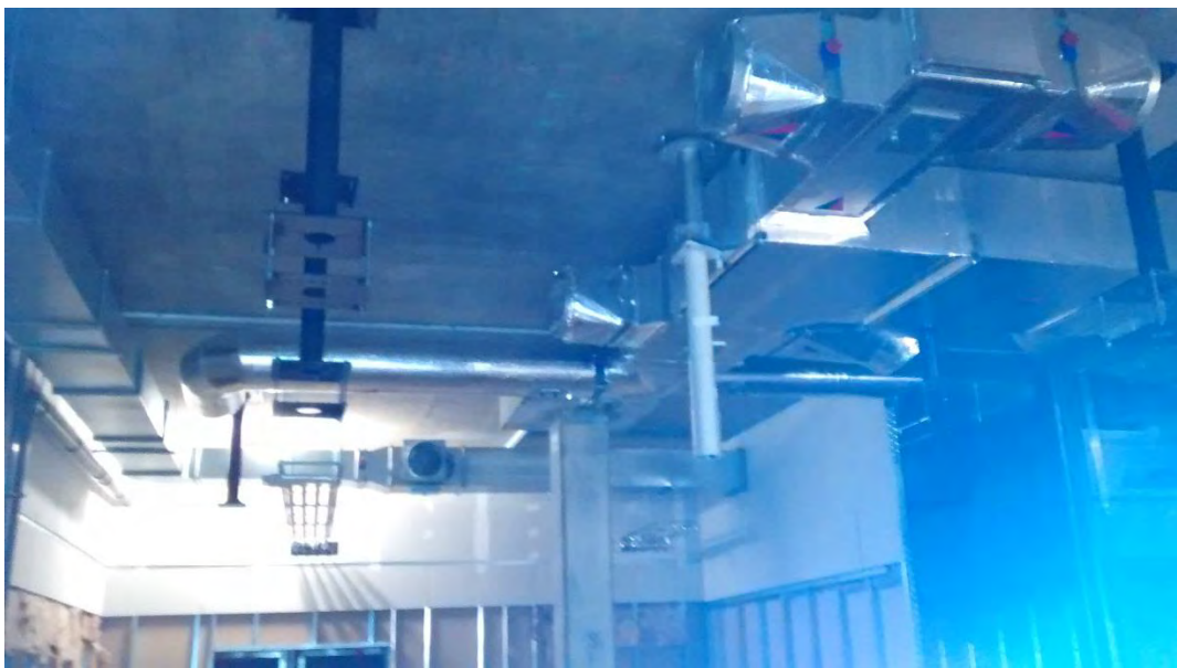
Fig 16 – Theatre Ventilation and Pendant Supports Level 1
