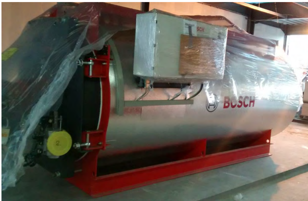
Fig 13 – One of Three Boilers in Energy Centre
