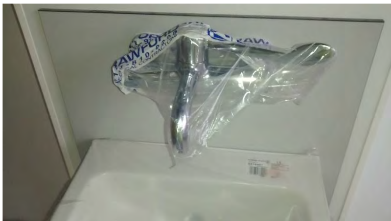
Fig 7 – Compliant Hand Basin and Hot and Cold Mixer Tap
