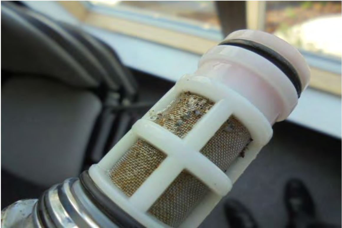
Fairly Extensive Contamination Observed on Markwik Inlet Filter
