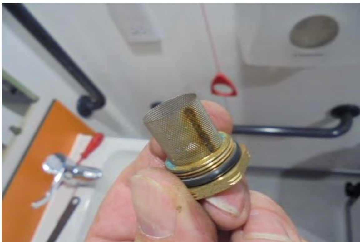
Significant Oxidation Contamination on Contour In-line Strainer
