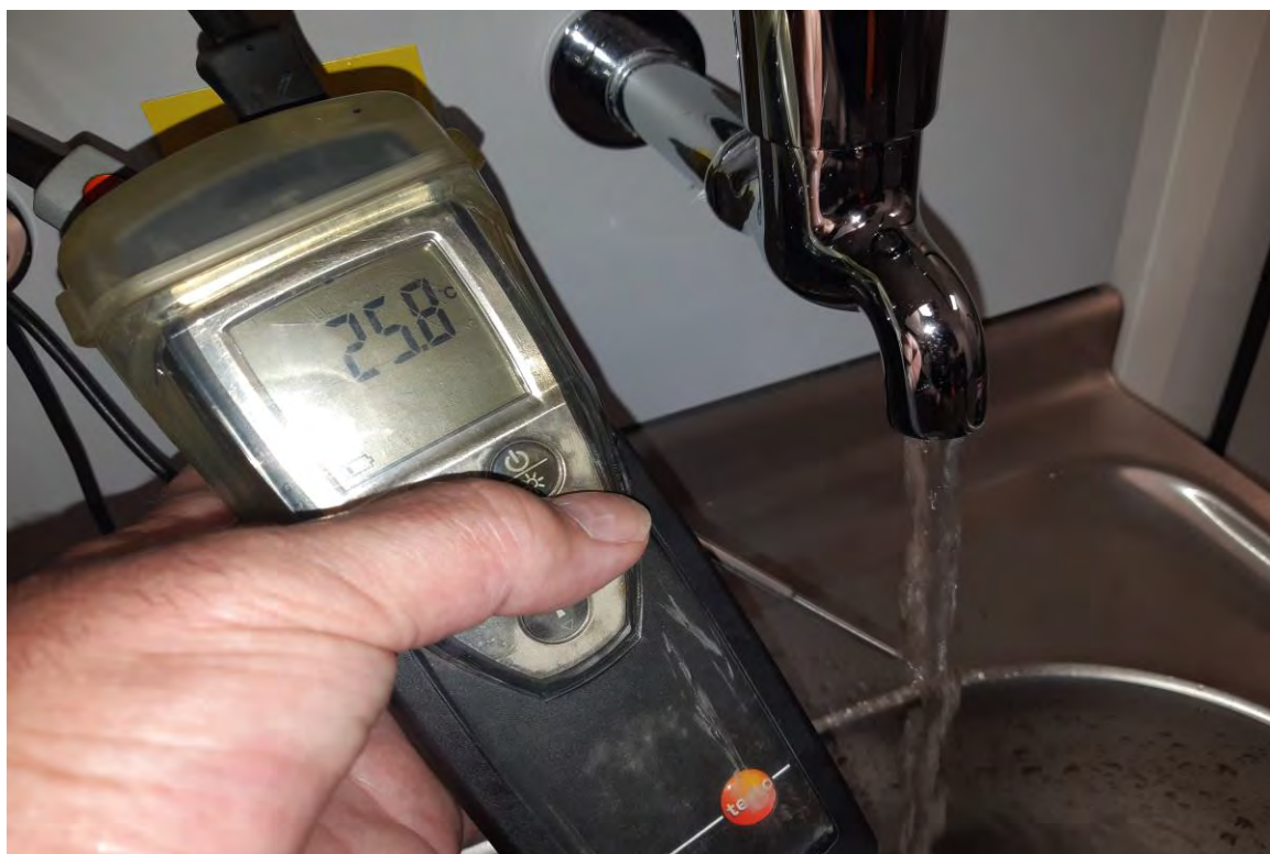
Elevated Cold Water Supply Temperature Recorded at End-of-Line Outlet
