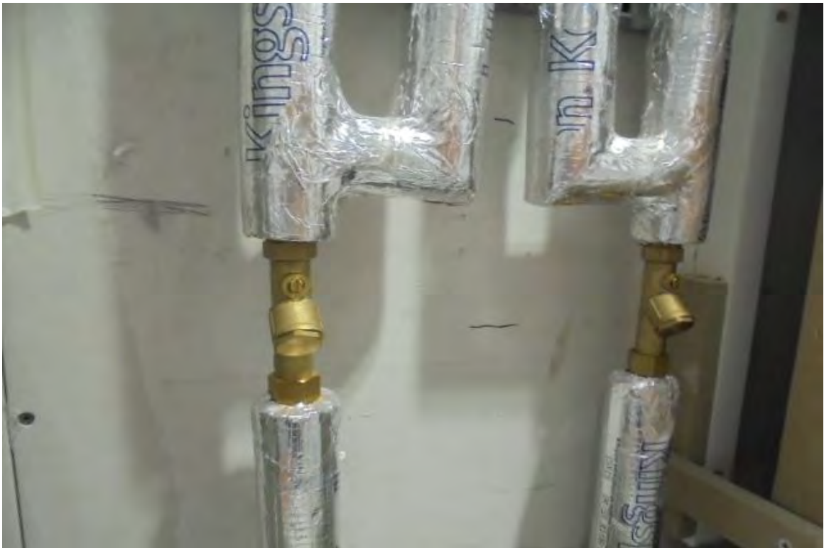
Hot and Cold Supplies to Contour Taps Provided With In-line Strainers
