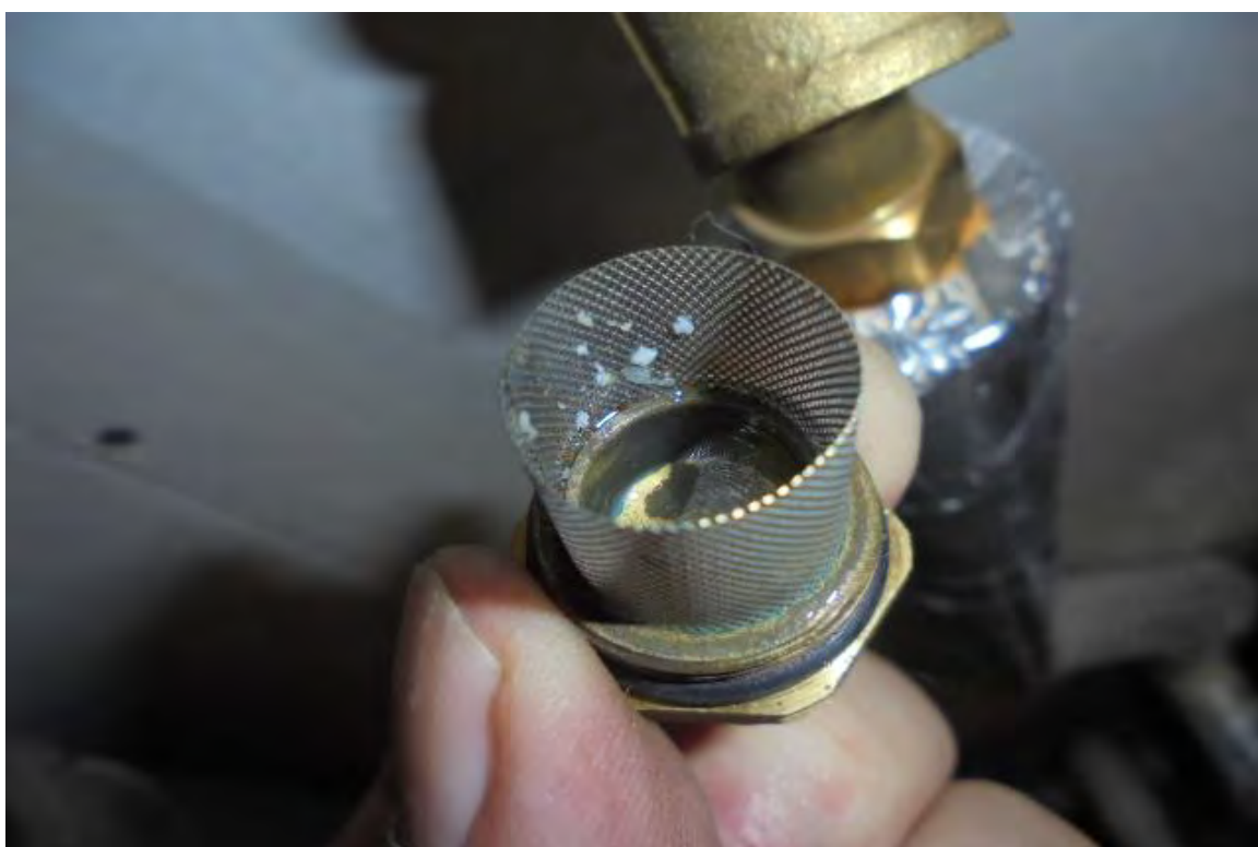
Installation Debris Retained in Contour In-line Strainer
