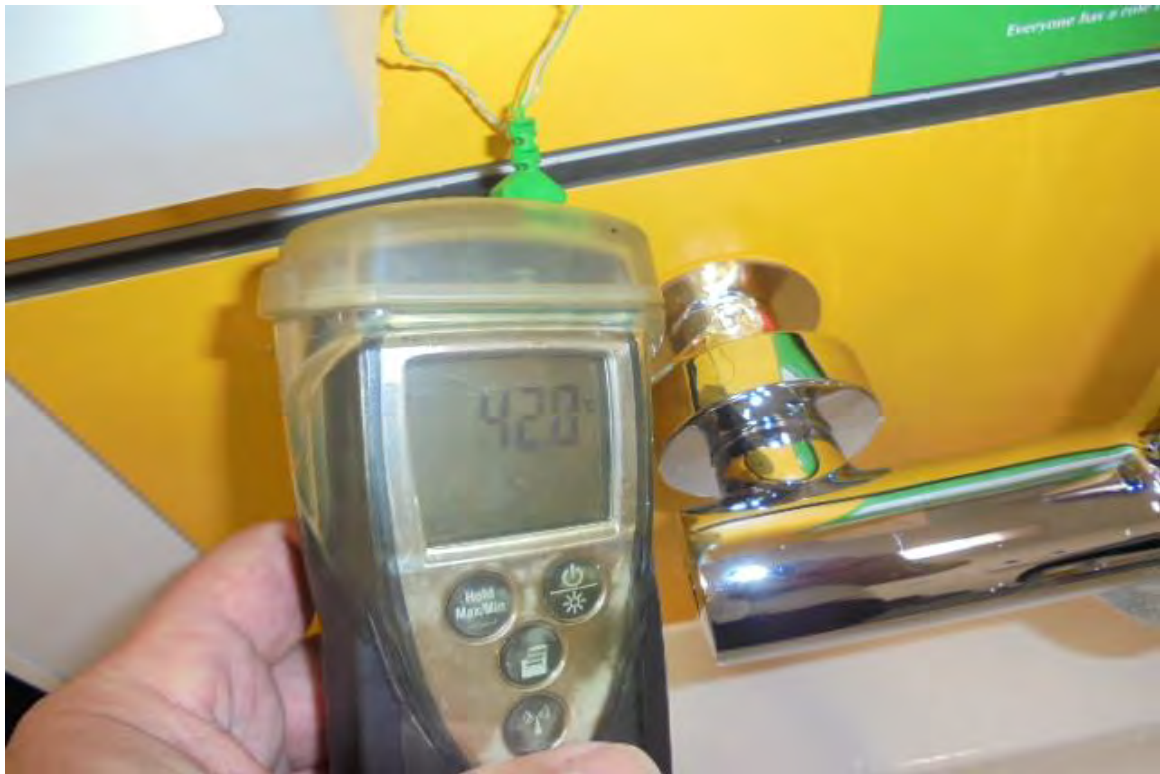
Low Hot Water Supply Temperature to Markwik Inlet
