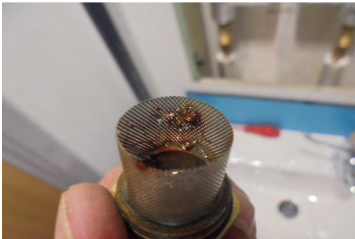
Substantial Debris Accumulation on Contour In-line Strainer
