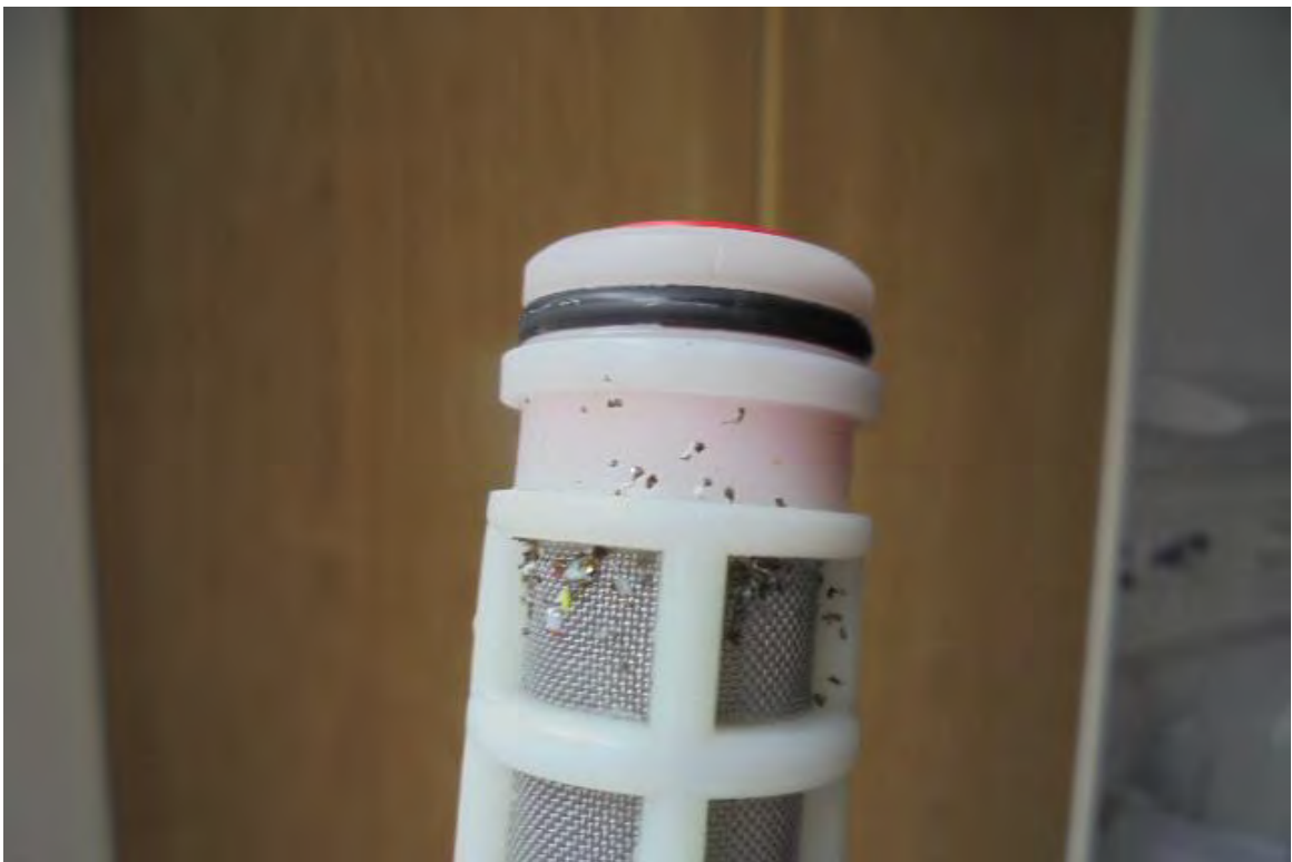
Installation Debris Accumulation on Markwik Inlet Filter
