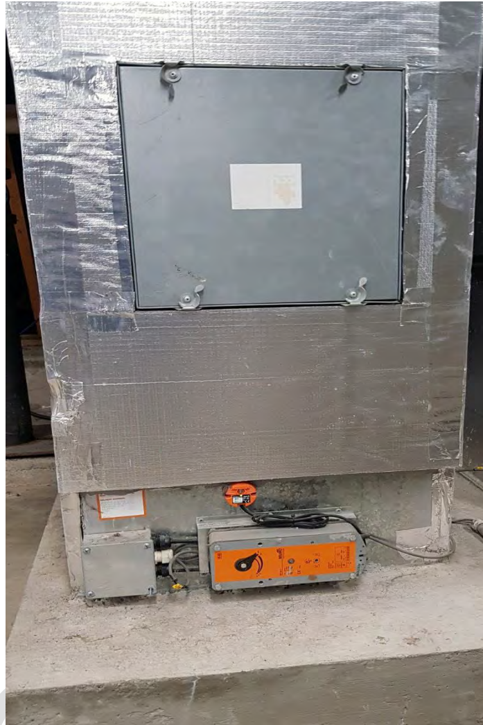
Figure 10 Fire damper with test switch and inspection hatch
