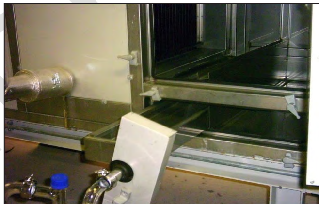
Figure 7 Removable AHU drainage tray
