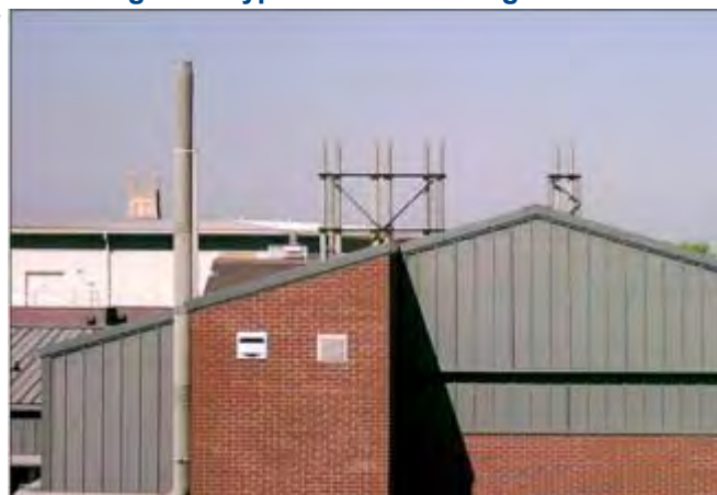
Figure 9 Typical LEV discharge stacks
