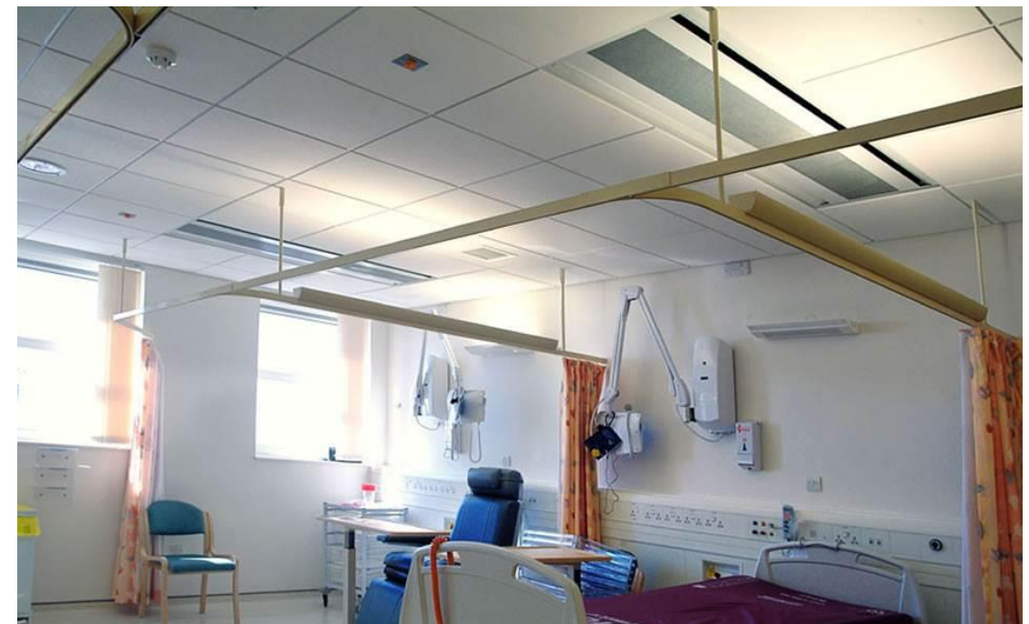
Patient environmental comfort is controlled locally by chilled beam
